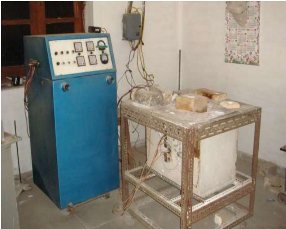
Figure 2.1 Global Furnace used for melting.
