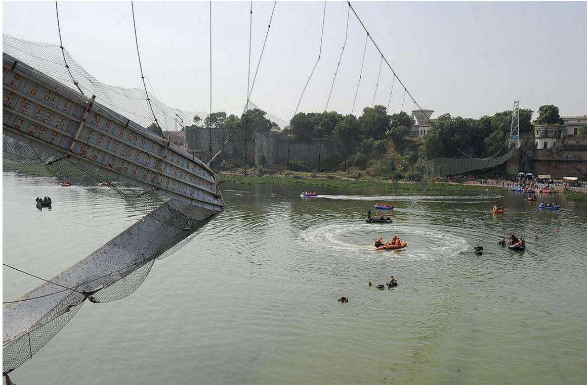
Figure 1.12: Collapsed pedestrian bridge, Morbi, Gujrat (The Hindu)
