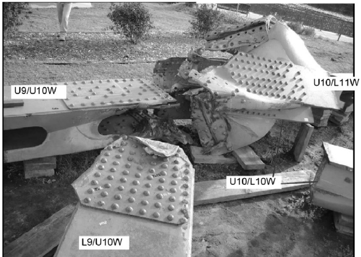
Figure 1.9: Gusset plate failure at joint U10 (Liao et al. 2011)
