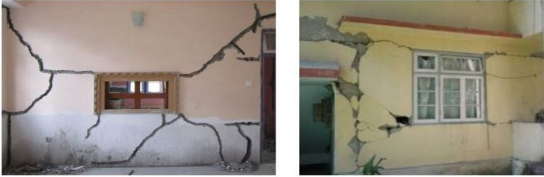
Figure 2.4: Typical damage to infill walls with openings observed during the 2011 M6.9 Sikkim earthquake [46]
