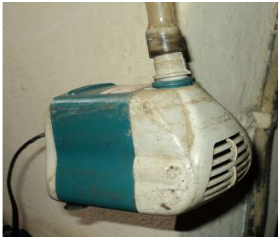
Fig. 3.11: Picture of Flushing Pump
