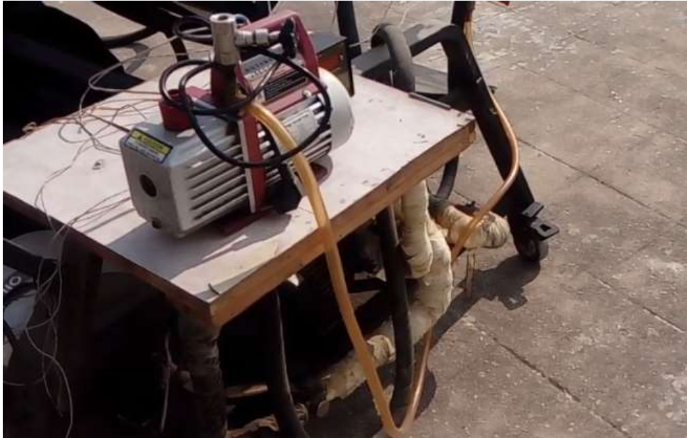
Figure 3.11: Photograph of vacuum vane rotary pump to create the vacuum at annulus
