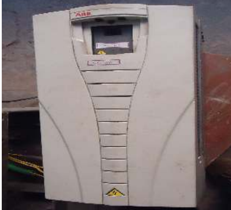
Figure 4.23: Variable Frequency Drive for 9.5 mm feedstock Continuous Extrusion setup
