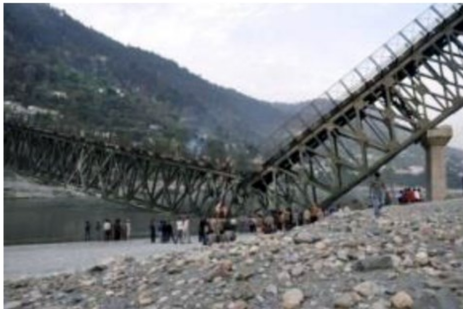
Figure 1.2 Failed Chauras bridge during casting of deck slab. [R. K. Garg et al. (2020)]
