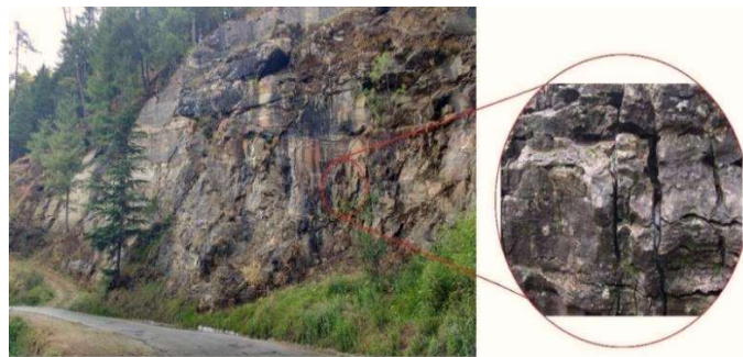
Fig. 4.7. Increased joint spacing (solution space) in calcareous rocks due to seepage
