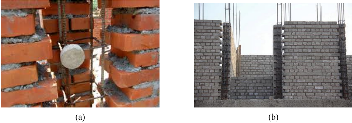
Figure 1.5: a. Typical construction sequence of a CBM wall, with concrete poured after masonry erection, and b. construction of a student hostel at IIT Gandhinagar [11]
