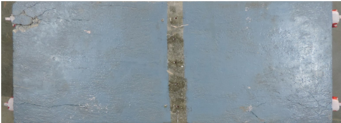
Figure 3.26: Deck slab top view after failure
