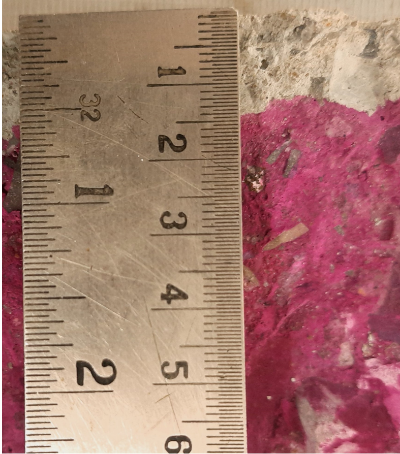
Figure 6.39: Carbonation depth of F100RC
