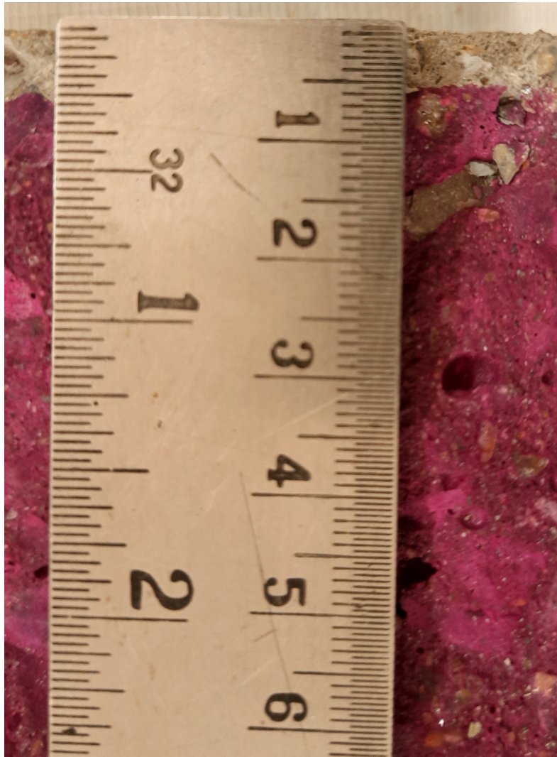
Figure 6.41: Carbonation depth of C60F60RC
