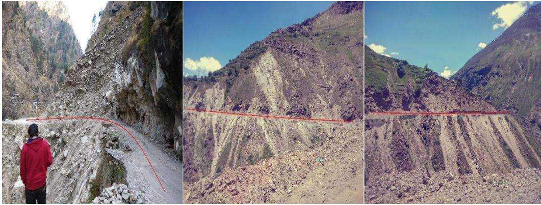
Fig. 2.2. Several localised slope failures are observed along the hill roads
