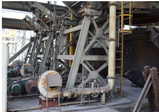
Figure : 5.1 Motor Mounted Centrifugal Blowers for the Burners
