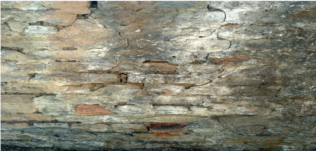
Figure 4.11 A view of cosmetic/hairline to minor cracks on brick-cement wall of another house at 300m from blast site.
