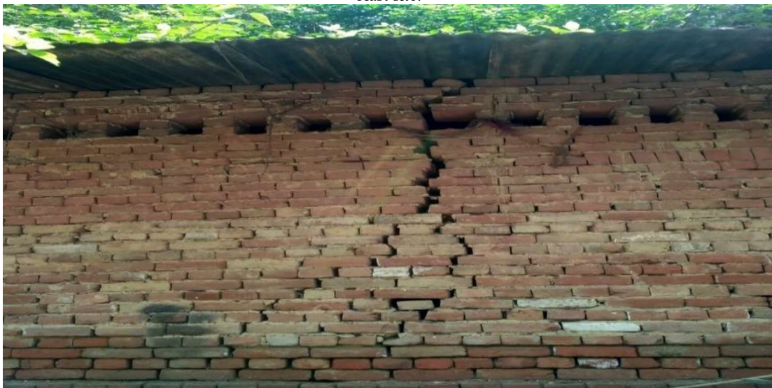
Figure 4.12 A view of minor to major cracks on the brick-mud mortar wall at 250m from blast site.
