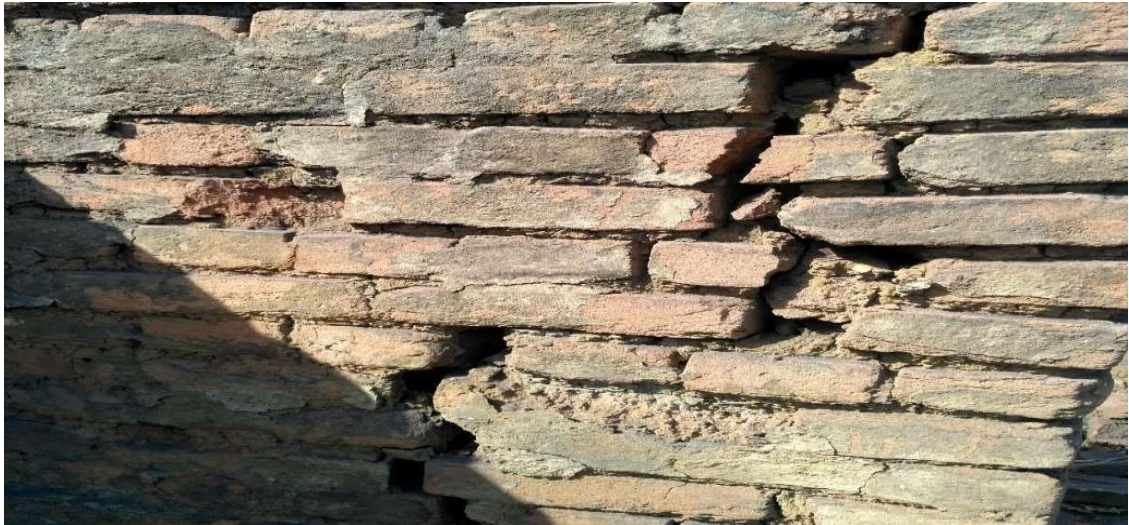
Figure 4.13 A view of major cracks on the non-plaster brick-mud mortar wall at 250m from blast site.
