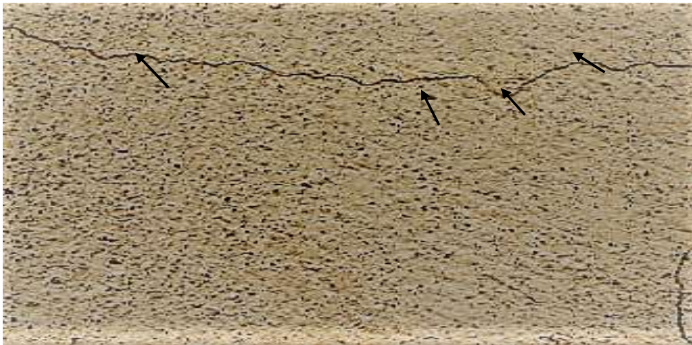
Figure 4.8 A view of cosmetic/hairline crack on the plaster wall at 200m from blast site.
