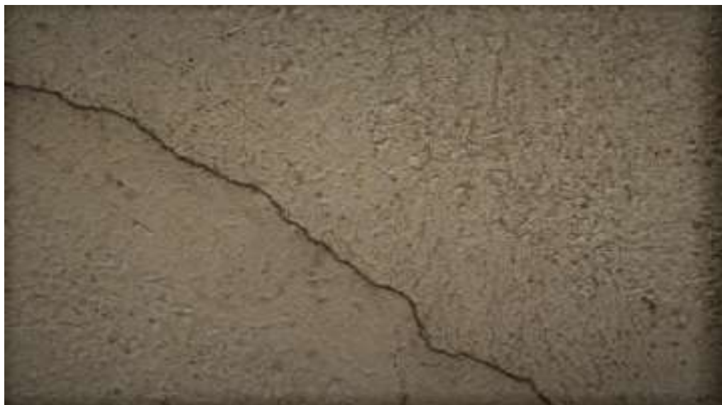
Figure 4.9 A view of minor crack on the plaster wall at 200m from blast site.
