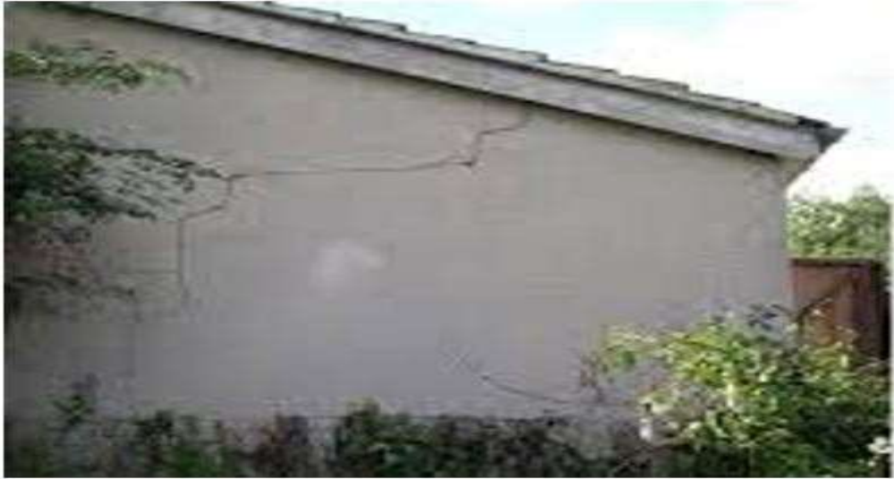
Figure 4.7 A view of cosmetic/hairline crack on the plaster wall at 200m from blast site.
