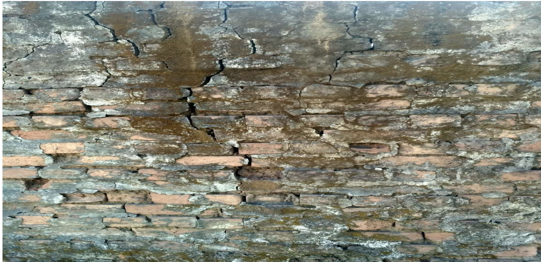
Figure 4.10 A view of cosmetic/hairline to minor cracks on brick-cement wall at 300m from blast site.
