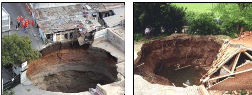
Figure 2.1 Danger to the life and property due to pot-hole (Lokhande et al. 2015)
