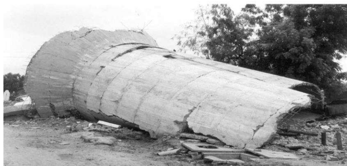
Fig. 2.2: Collapsed 265 kL water tank in Chobari village about 20 km from the epicenter. [Rai, 2003]
