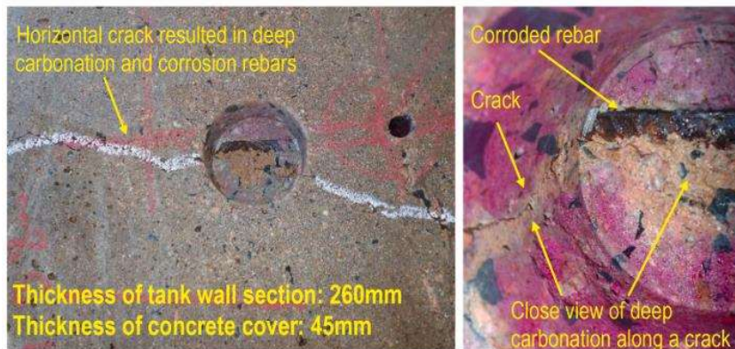
Fig. 2.5: Horizontal cracks resulting in corrosion of rebars [Rodd and Castel, 2022]
