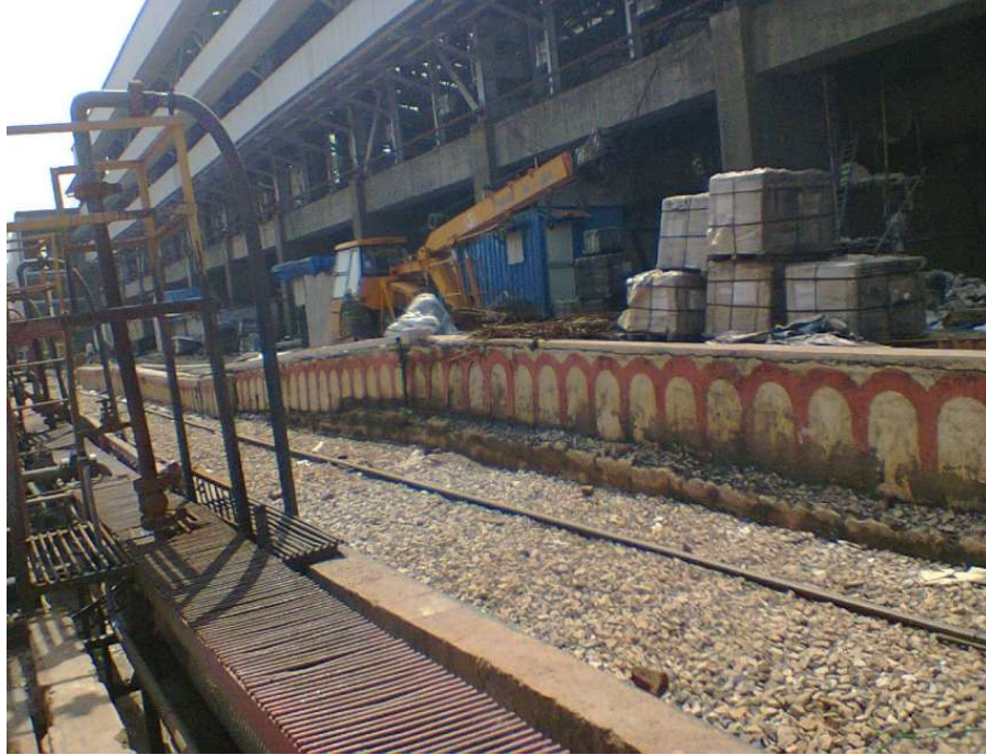
Figure 1.4: Heaving in wall of railway platform of aluminium plant due to alkali interaction
