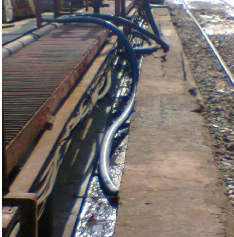
Figure 1.3: Leakage of alkali solution during unloading in an aluminium plant
