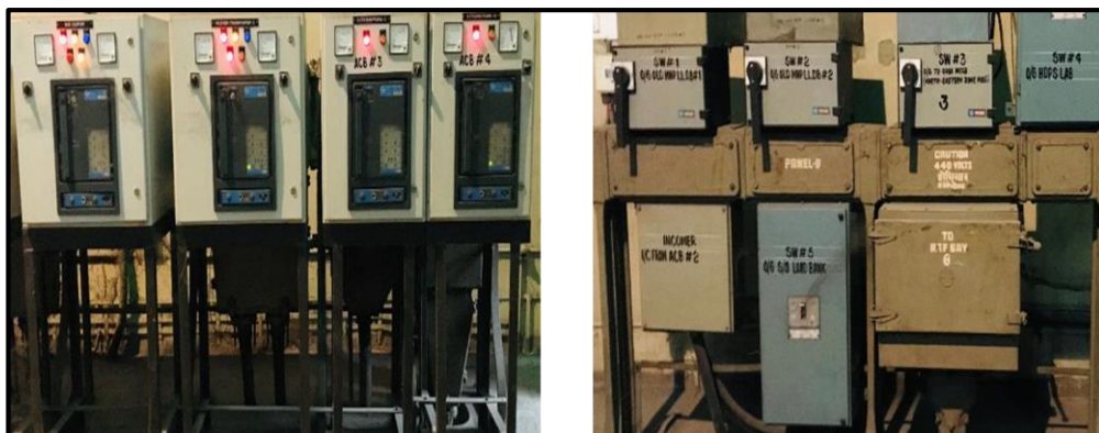
Figure 6.7- (a) and (b) Sub distribution panels considered for solar installation
