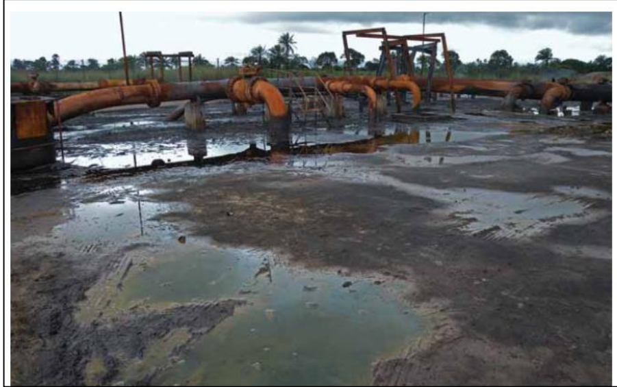
Fig. 1.5 A view of contaminated site at Bomu station due to severe spillage (Image source:www.google.com)
