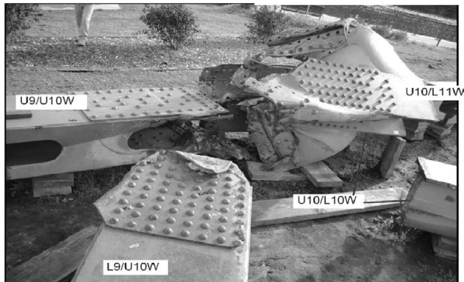
Figure 3.2 Failure of gusset plate at U10 (M. Liao, et. al. , 2011)
